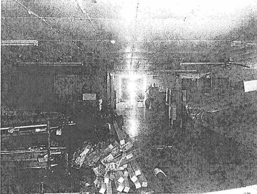
Picture taken April 28, 2022; Building materials stored in the interior of the structure for renovations.
