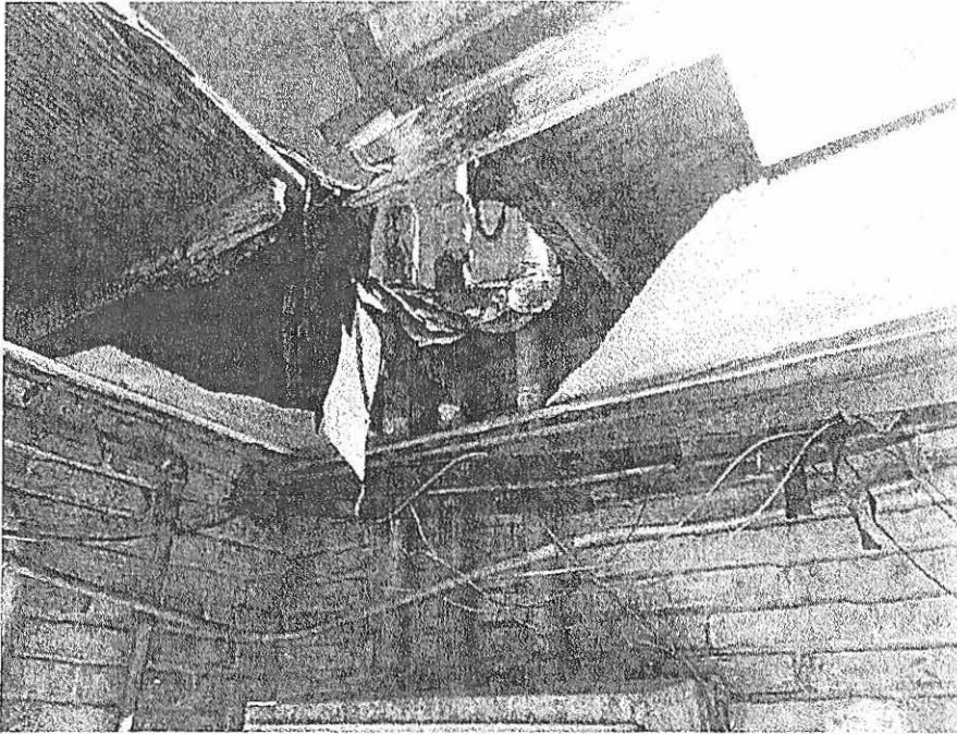
Picture taken April 28, 2022; fascia, soffit and roof severely rotten from damaged roof, allowing moisture on to the electrical boxes possibly causing damage the electrical supply to the building.
