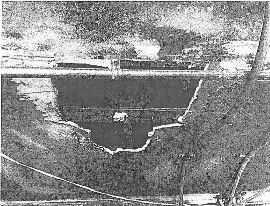
Picture taken April 28, 2022; roofing severely rotten and damaged from water, mold present throughout in equipment room.
